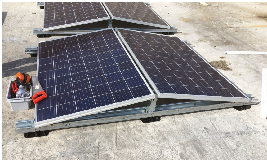
Back-to-back roof mounted PV panels
